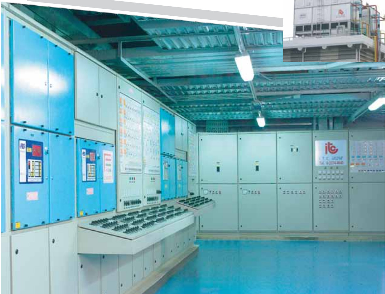
Evaporator Control Panel
