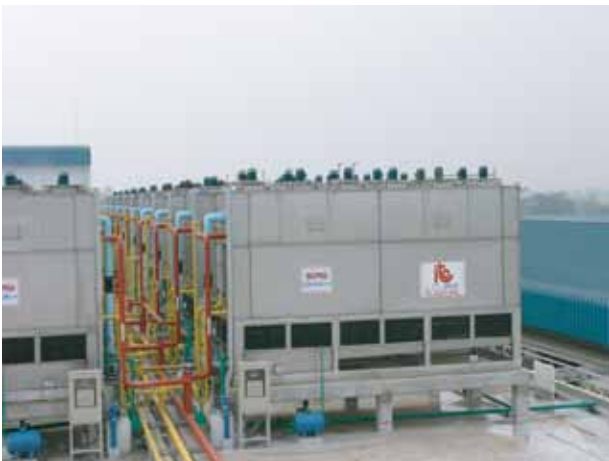
Photo 3 : Stainless Steel Evaporative Condenser.
