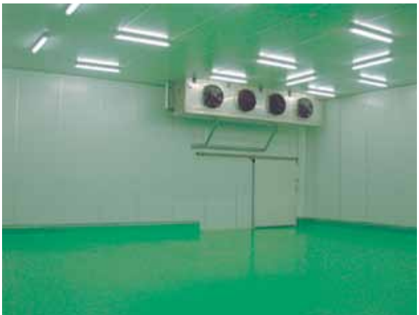
Photo 9 : Stainless Steel Unit Coller.
