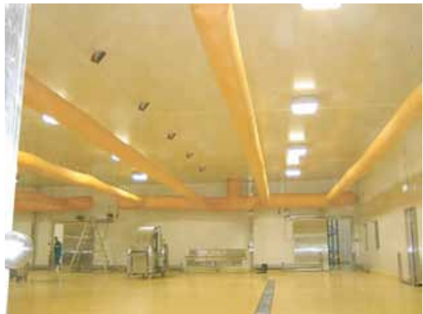
Photo 12 : +10 °C Air Sock (Low draft) Air Distribution.
