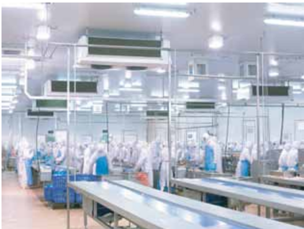
Photo 11 : 10 °C Low draft Unit Cooler.
