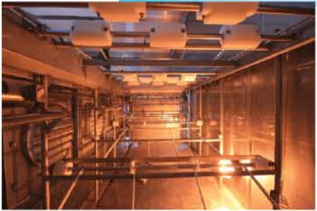
Multi-set fan section located under the conveyor belt
