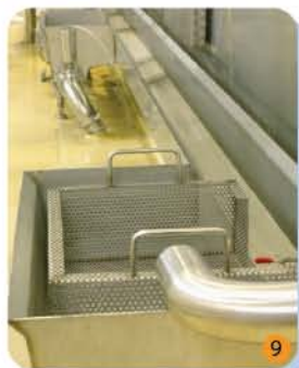
Recirculation type CIP system
