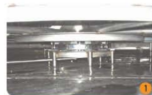
Bottom main bearing of Spiral drum
