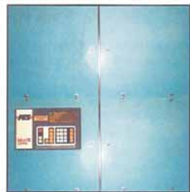
Double Height Enclosure with up to 4 I/O Racks
